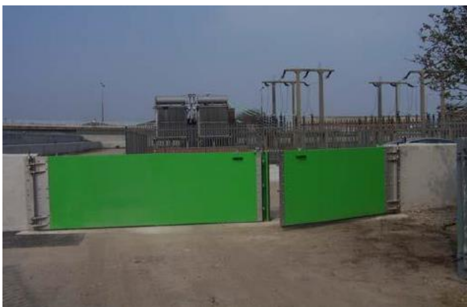
Figure 6.6: Flood protection gates (ENA ETR138 Annex 1)
